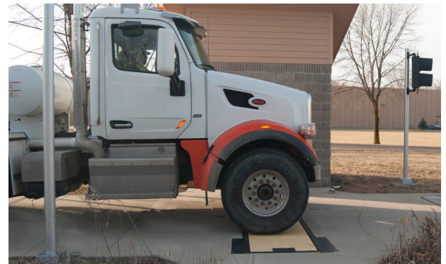
The LS-WIM System can be operated without the need for a gate operator. The driver is responsible for entering a code, or using a key fob to activate the system.
